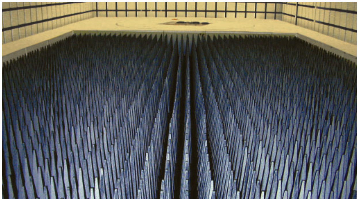
Antenna Measurement Facility with Floor Absorber Detail
